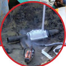
6" Pipe Freeze on DI Water Line
